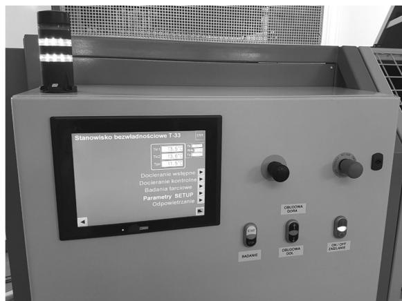
Fig. 4. Control cabinet integrated with the T-33 dynamometer
